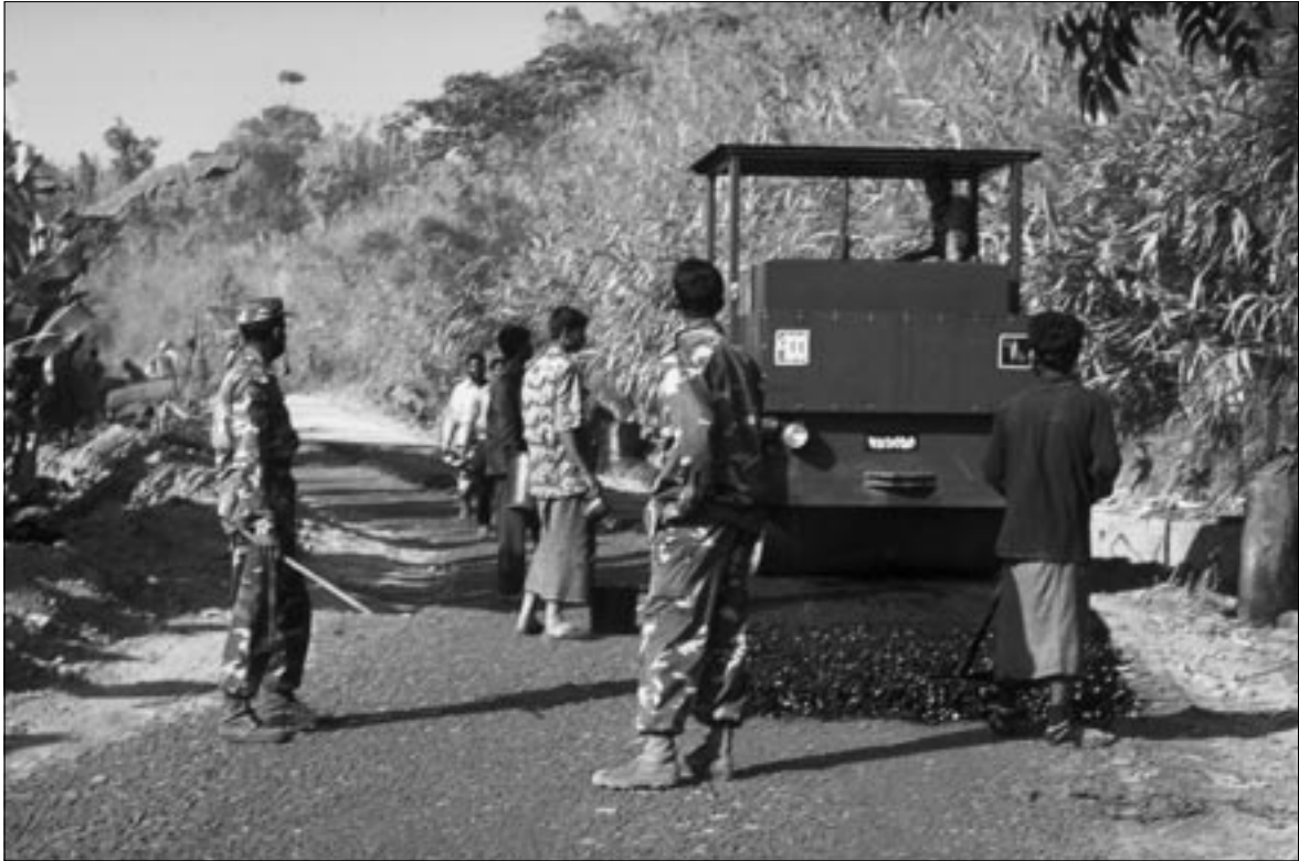
Road construction between Chimbook and Thanchhi, Bandarban District, by the army and Bengali workers
